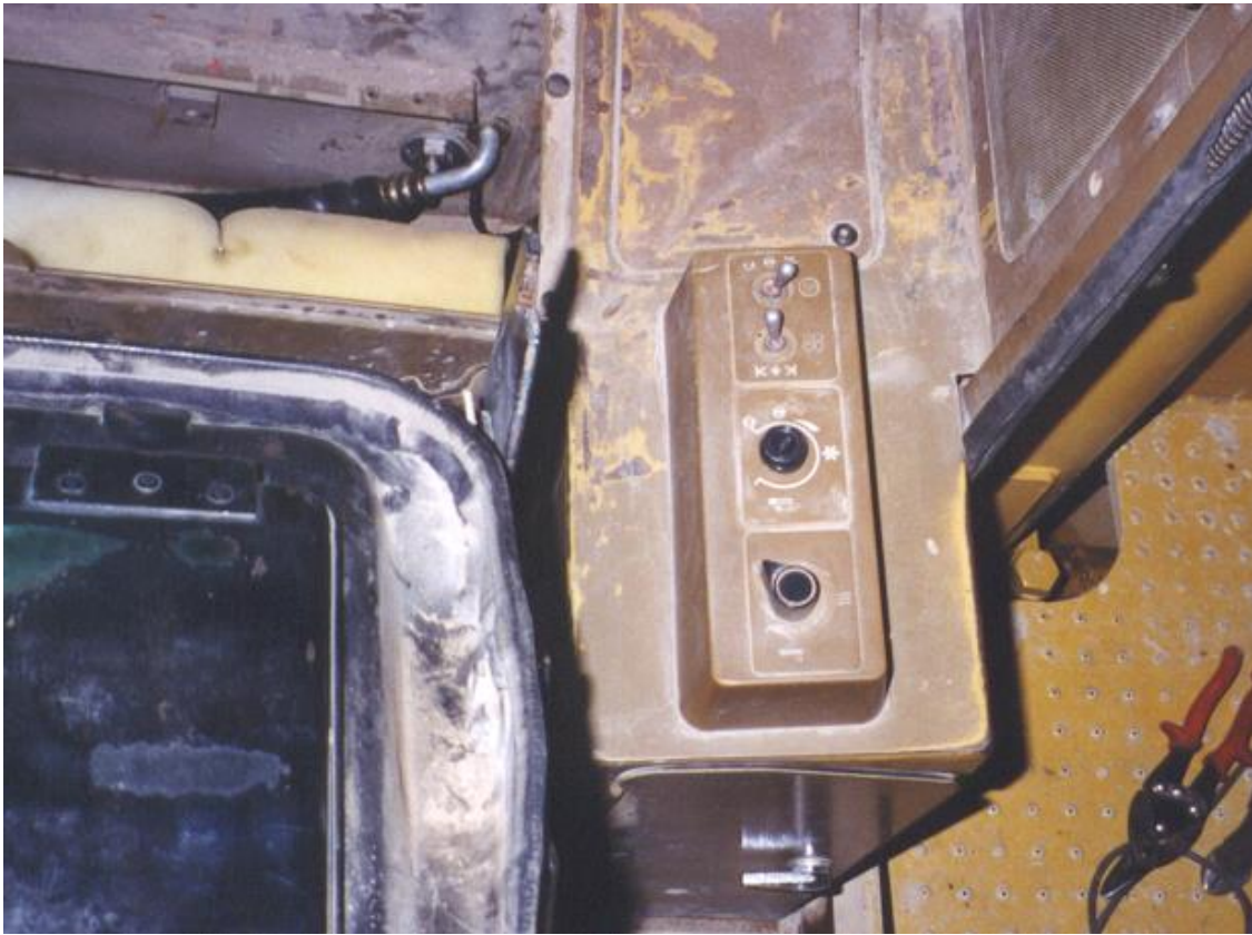
Thermostat in position.
